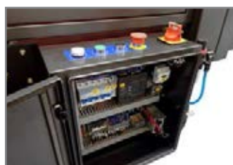
PANNELLO DI CONTROLLO CON PLC CONTROL PANEL WITH PLC
